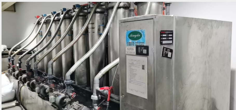
Water Recycling System
